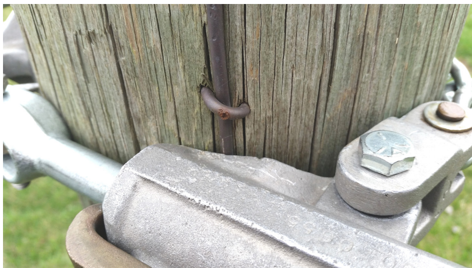
Current Chance Cluster Bar (T6001549) in conductive contact with bare pole ground with staples
